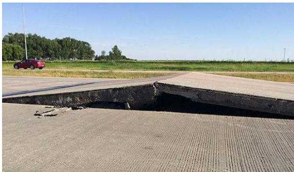
Concrete road 'buckling' due to heat. Image from: http://www.accuweather.com/en/weather-news/roads-buckle-shatter-in-central-us-amid-june-heat-waves/58223451
