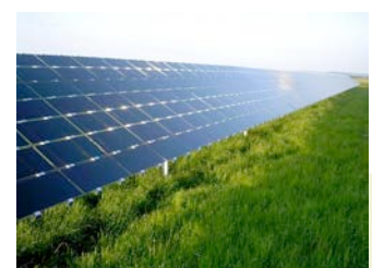
Thin film solar panels
